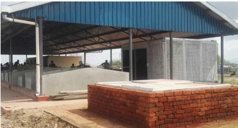
Fig. 25: Zero energy brick cooler and charcoal cooler at Kalobeyei Market in Turkana County
