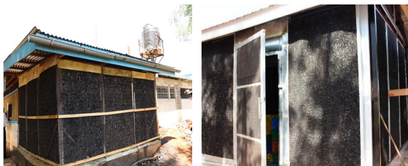
Fig. 14: The original charcoal with a wooden frame and the improved version with galvanized aluminium frame
