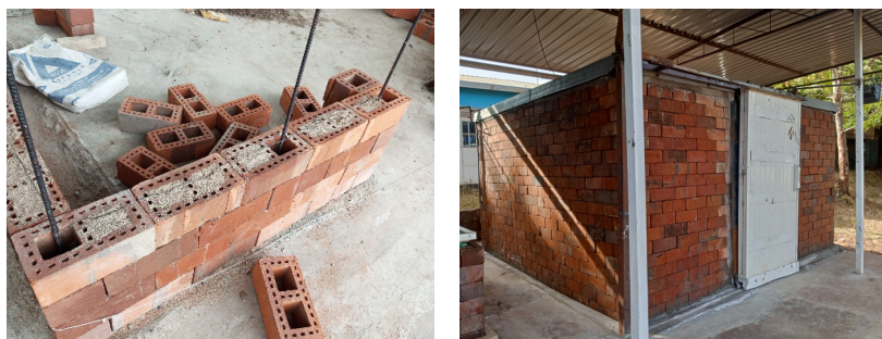
Fig. 13: The Resized ZEBC – under construction and the finished product at Cold Storage Tech Hub
